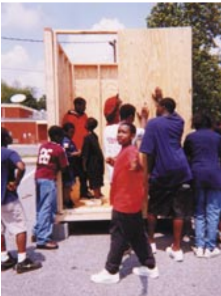
The panels completed, the young construction workers get to see the hut go up.
